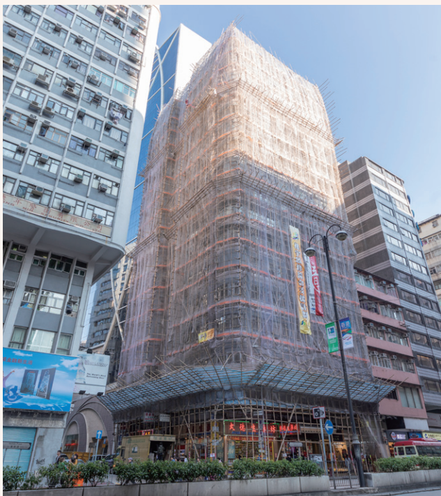
百樂大廈的復修工程接近完成。 The Pak Lok Building's rehabilitation work is near completion.
